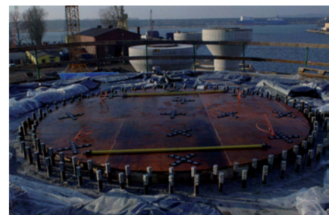
Fig. 9: Position of the mounting bolts in the concrete foundation and preparations for the measurement
